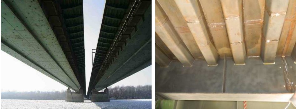
Fig. 1. The Grot-Rowecki Bridge: general view of box girders (left), the orthotropic deck (right)
