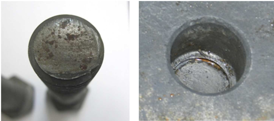
Fig. 5. The brittle fracture surface of bolt and a hole with end of bolt
