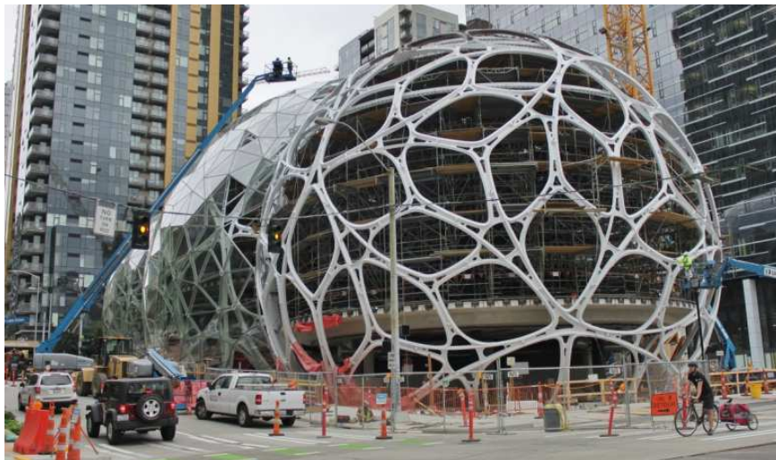
Fig. 6. Amazon Spheres – spherical conservatories serve as employee lounge and workspace located on the headquarters campus of Amazon company in Seattle, USA, completed in January 2018: steel structure under construction (author of photography: SounderBruce [9])
